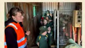
Having a look at the generator, which is currently out of action.
